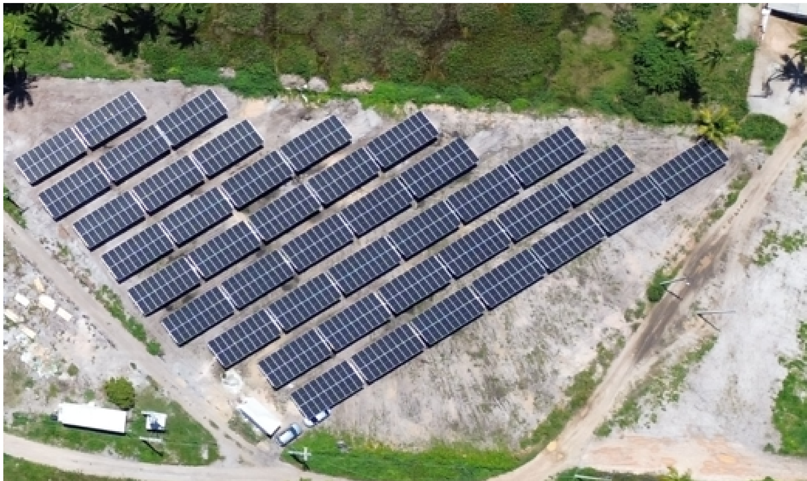
Pousada Camurim Grande 410,70 kWp - Maragogi/AL
